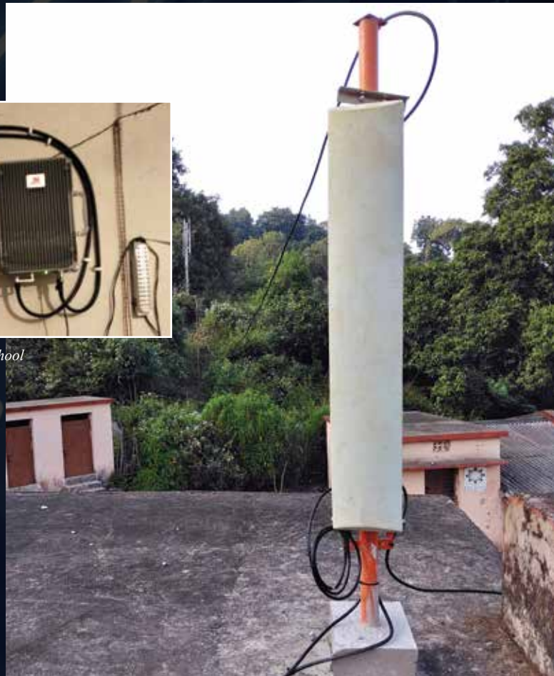
2-Port GSM antenna fixed on the 3 metre pole on the school rooftop.
