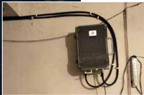
Repeater installed inside the school in Tamangi village (Odhisa).
